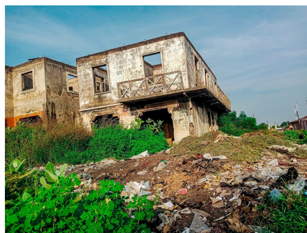
Plate 1. Abandoned burnt structure and debris after 2014 Wukari Crisis
